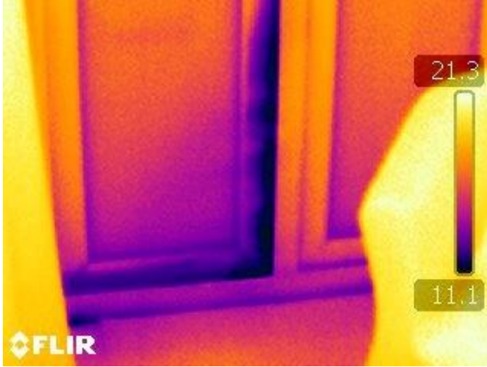
Fig 4 Example thermal image showing dark (cold) areas where there is cold air ingress around the surround of the doorway which leads outside.
